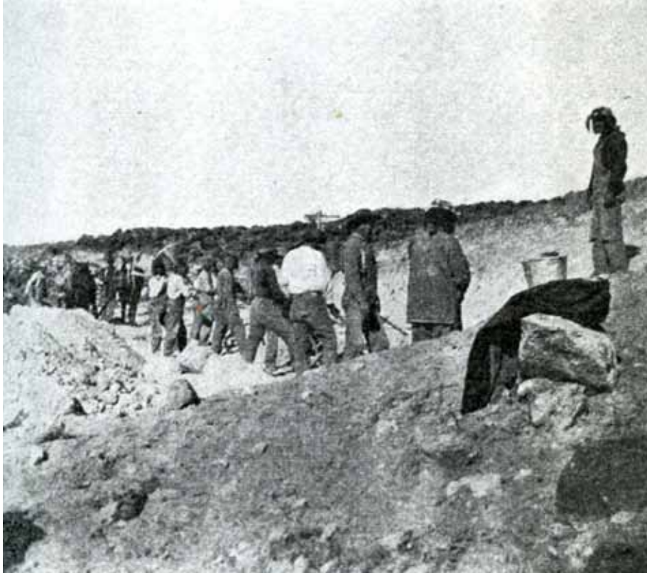
Men from Cochiti Pueblo providing local labor for La Bajada Hill road construction. (Sullivan 1909-1910: 181).
